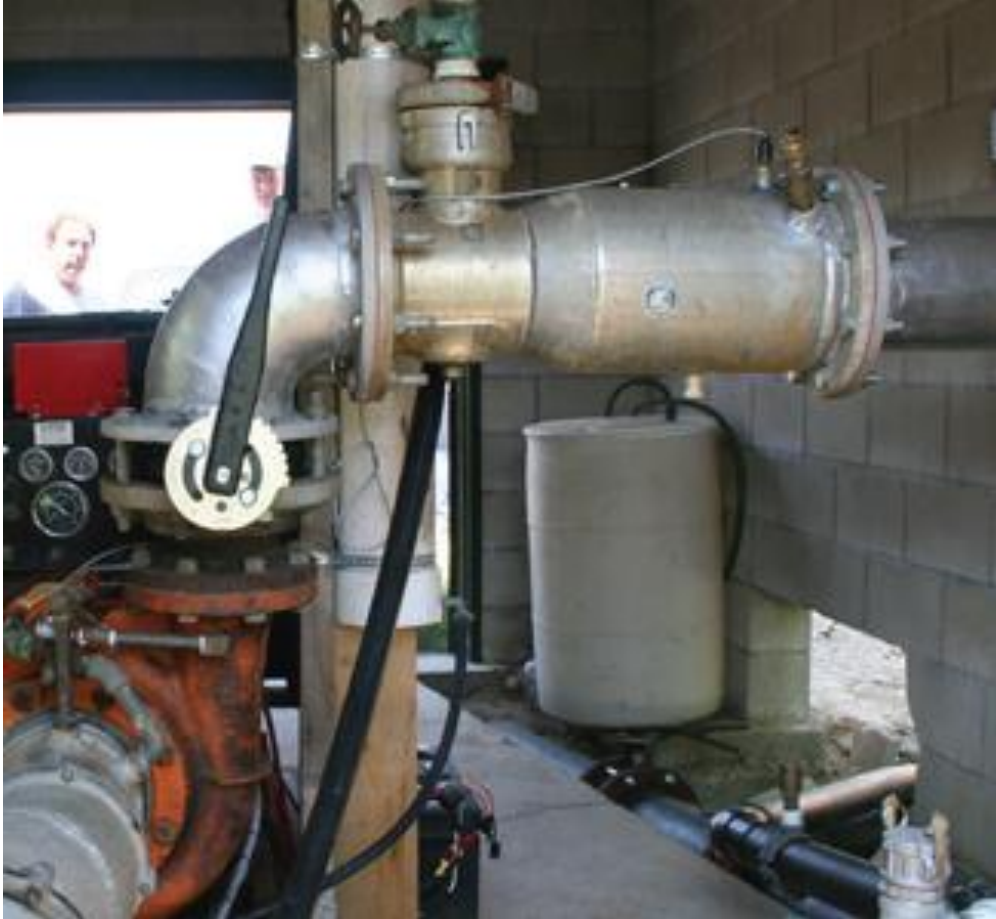
Figure 2. Centrifugal pump mounted on steel pipe. Credit USDA NRCS.
