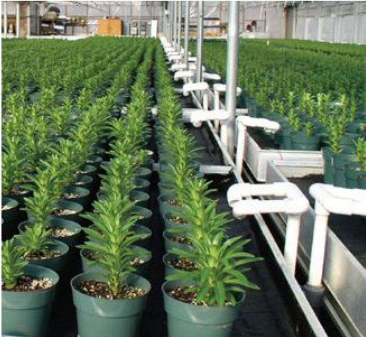
Figure 1. White PVC pipe in Ebb and Flood system. Credit USDA NRCS.
